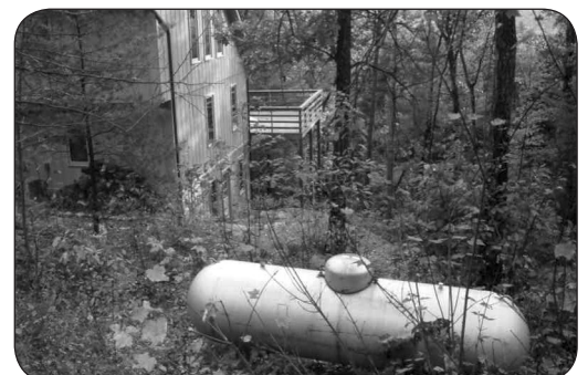
Propane is stored in a large tank. It is used to provide energy for heating, cooking, and drying clothes.
